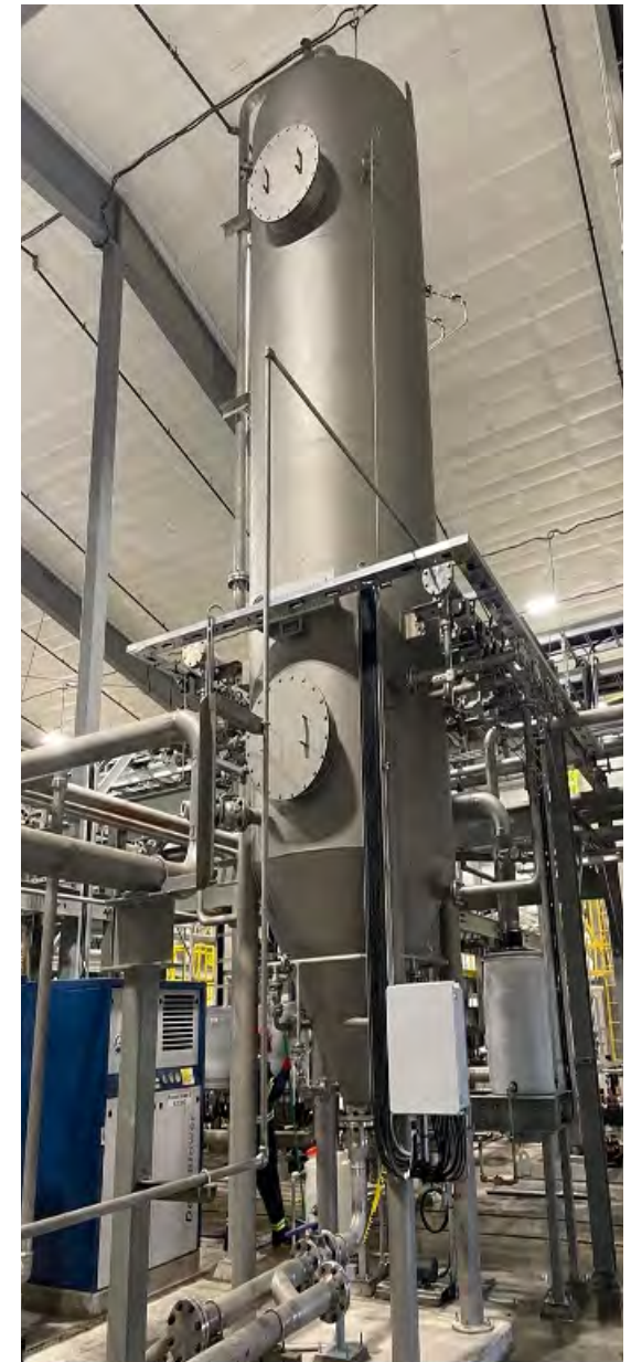
Sulfur Mitigation System YORKTON, SK, CANADA
